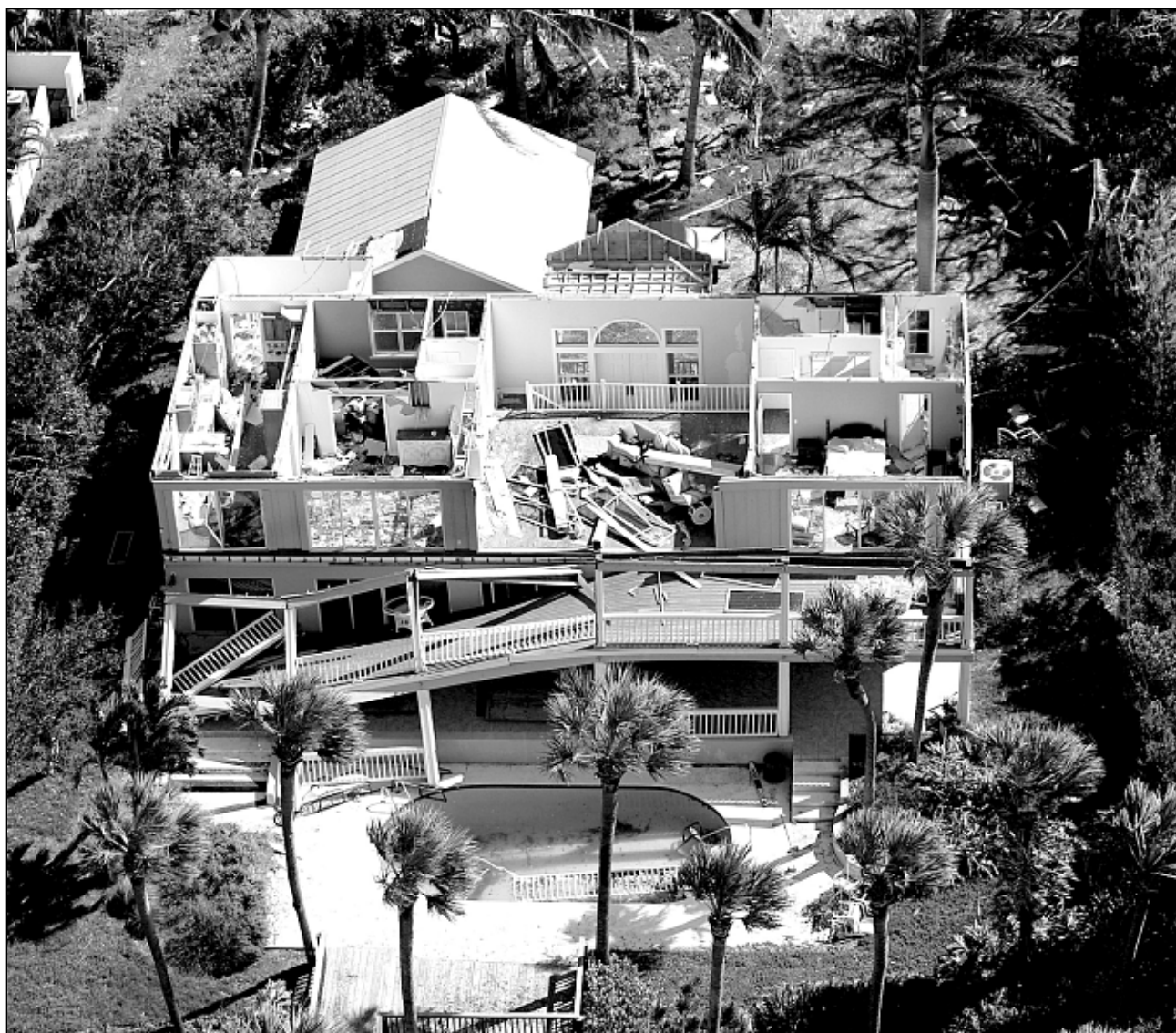
Hurricane Wilma tore the roof off this home on the St. Lucie River in Sewall's Point. State Chief Financial Officer Tom Gallagher warned that Wilma will affect insurance rates.
